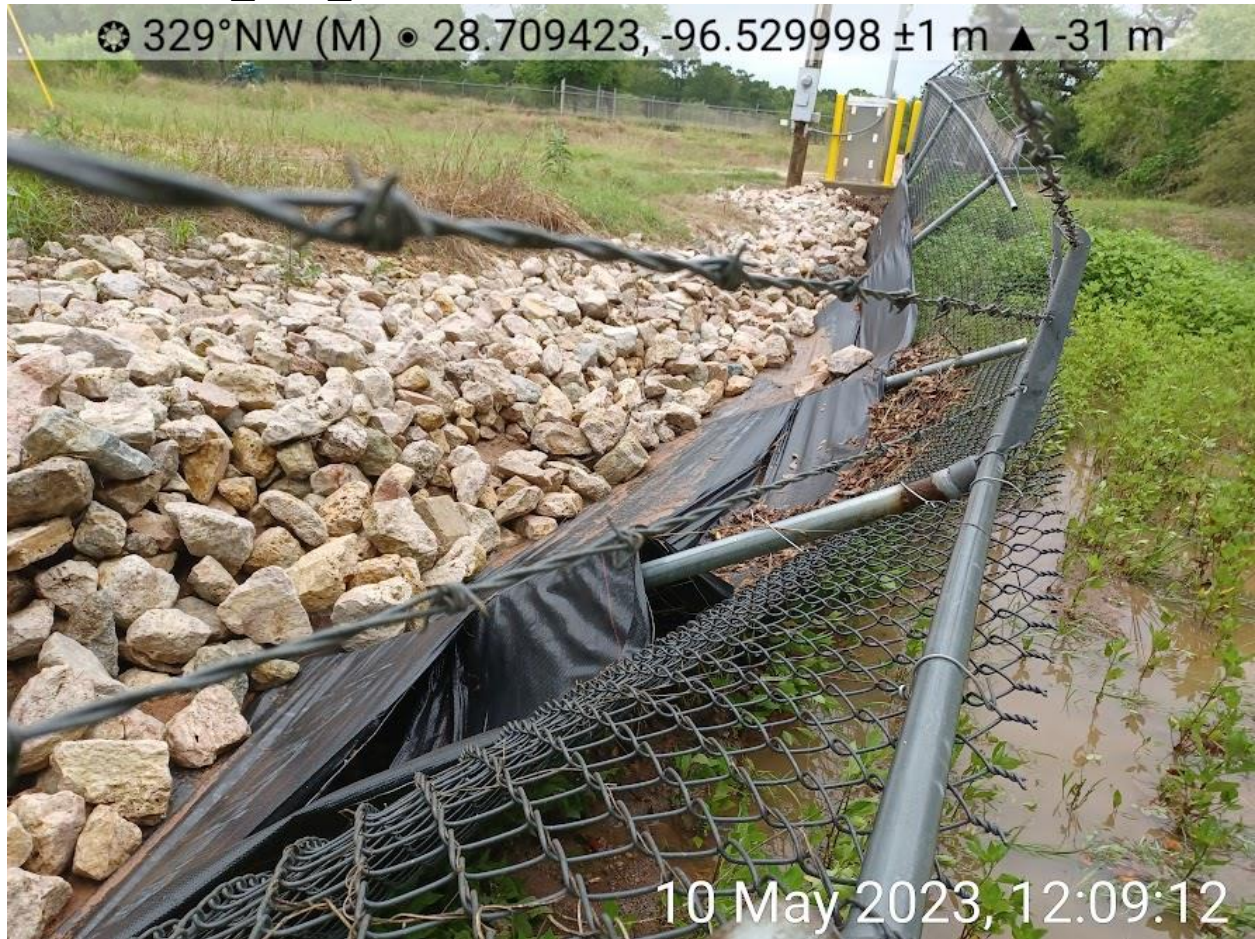
Fence line south of Outfall 014 laid over due to water flow.
