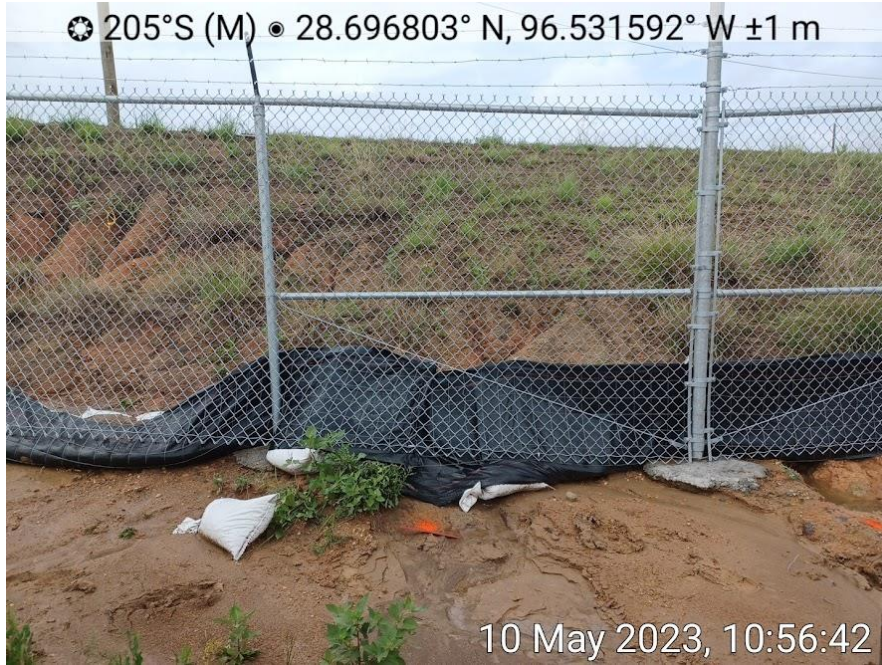
Silt fence adjacent to the flow reducers at Outfall 008. Silt fence was blown out due to flow, sandbags were washed under silt fence as a result of the damage.
