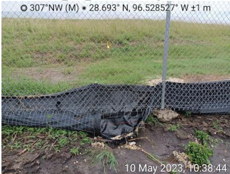
Silt fence North of Outfall 007 was washed out during recent rains.
